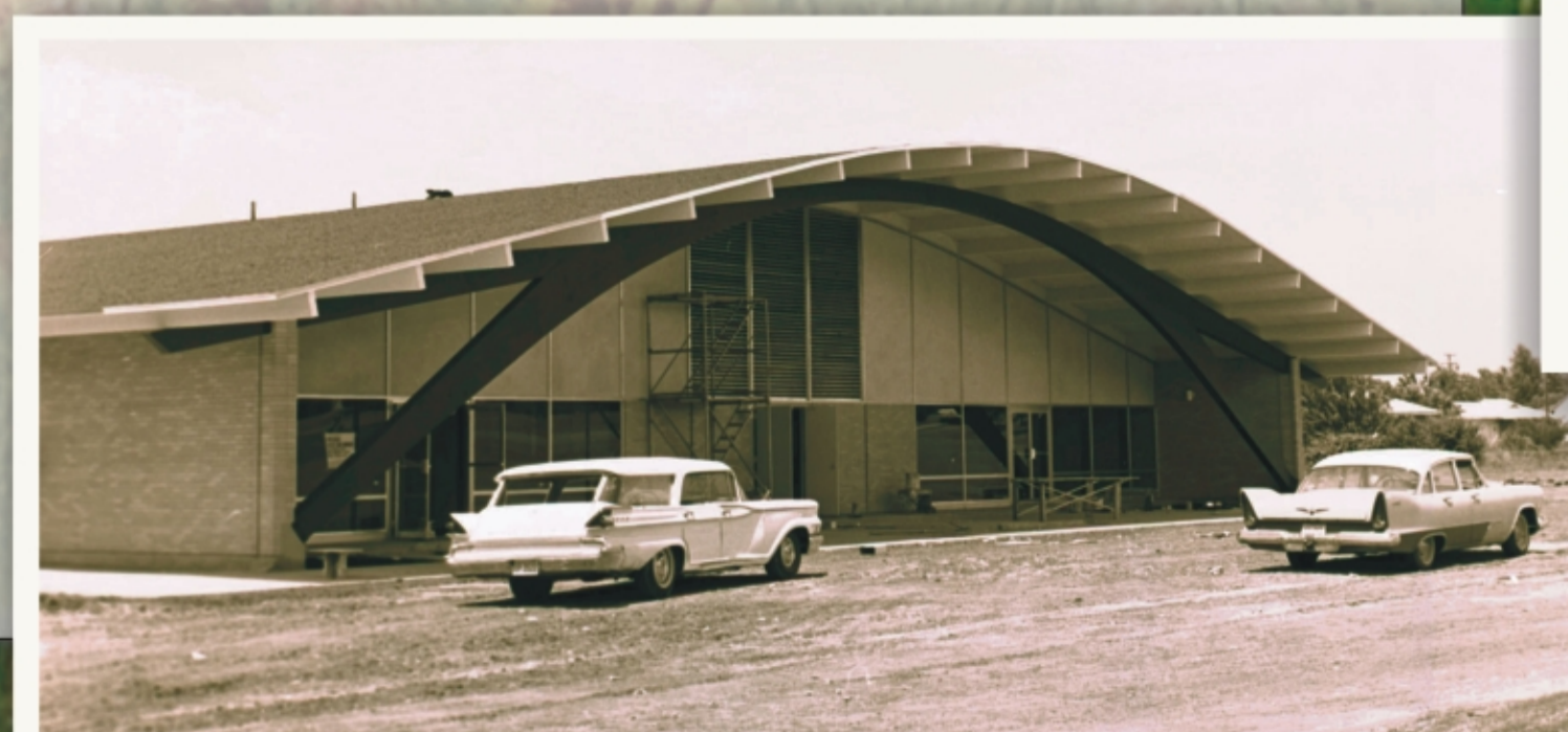
Near Completion - Construction is reaching final stages at the Arlington Recreation Center in Meadowbrook Park. J.J. Thomas Construction Company of Fort Worth is general contractor and Jarvis, Putty & Jarvis of Dallas are Architects for the facility. Noted in the Fort Worth Star-Telegram, June 29, 1963. Photo courtesy, Fort Worth Star-Telegram Collection, Special Collections, UTA Library, Arlington, Texas.
